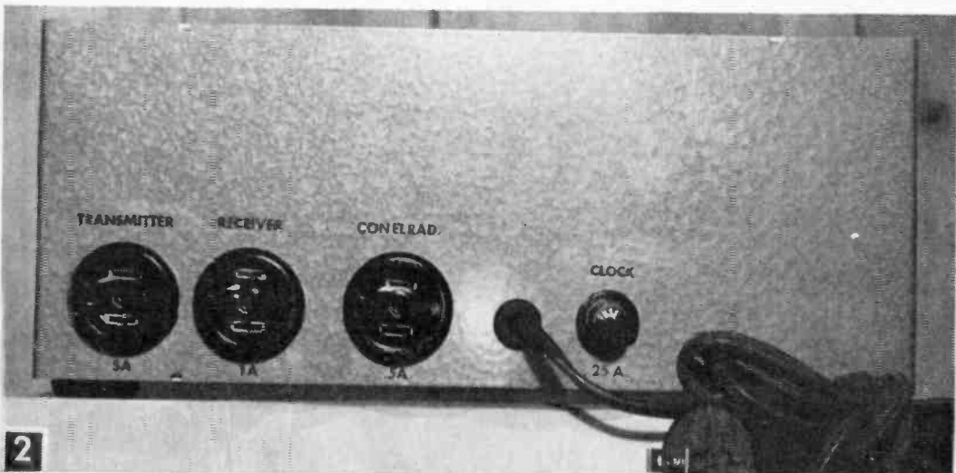
Rear view of power distribution center. If additional outlets are desired, slight relocation of the clock fuse and ac cord entrance will provide space for them.
